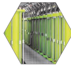
Flywheel energy storage
